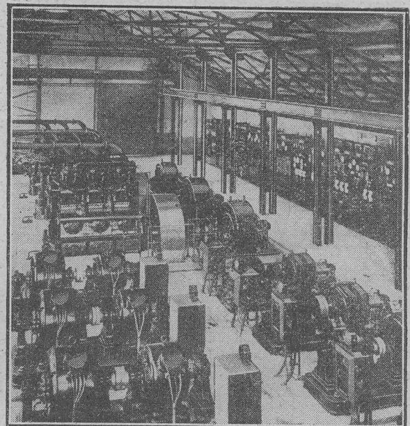
Generators and switchboards at the new G.P.O. beam station at Bodmin, Cornwall.
